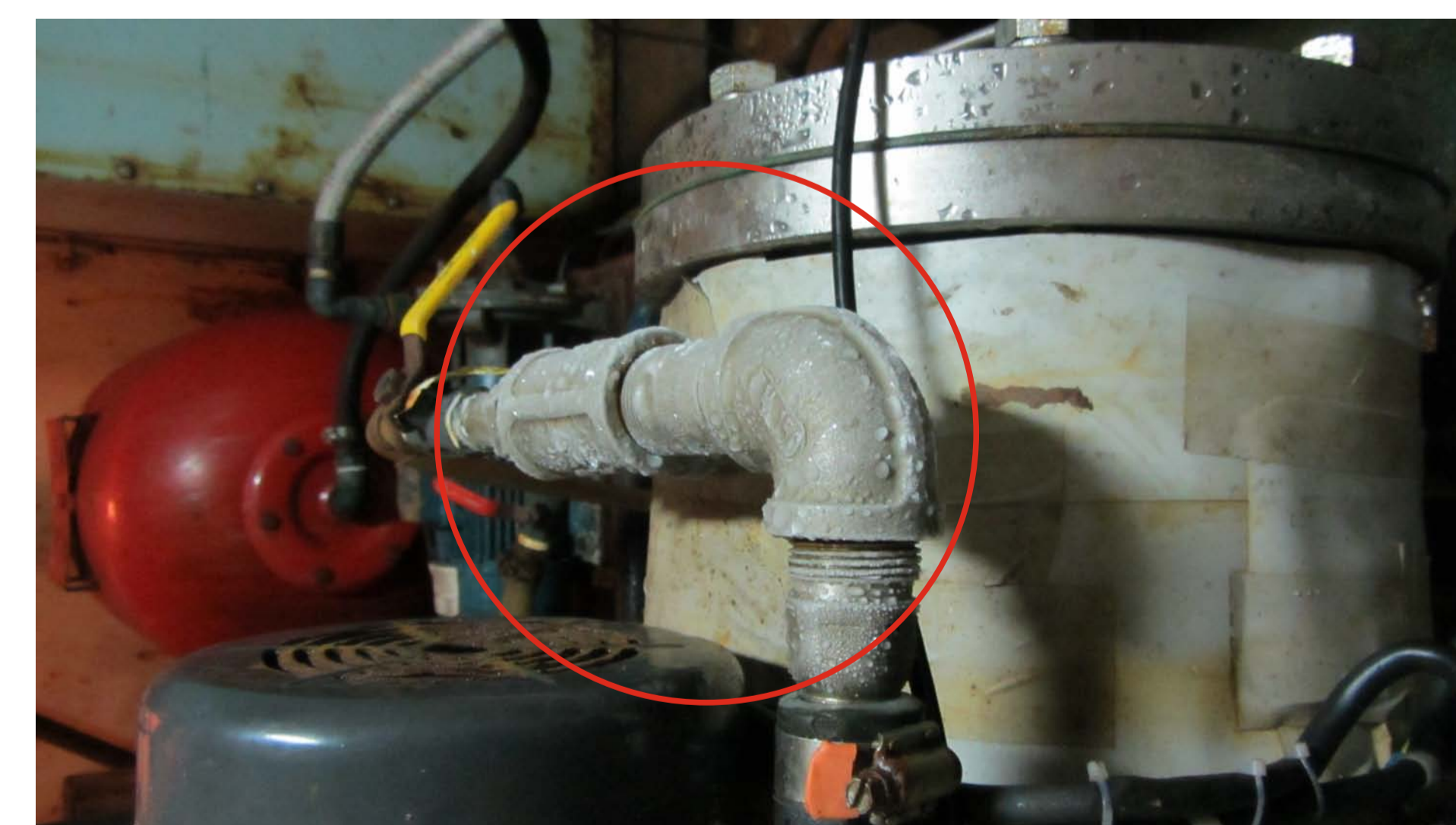
the Bellingshausen Sea conditioned the operation of the SSV due to the low water temperatures, which even caused that parts of the pump reached the freezing point and the intermittent stopping of the sensor. (See photo).
