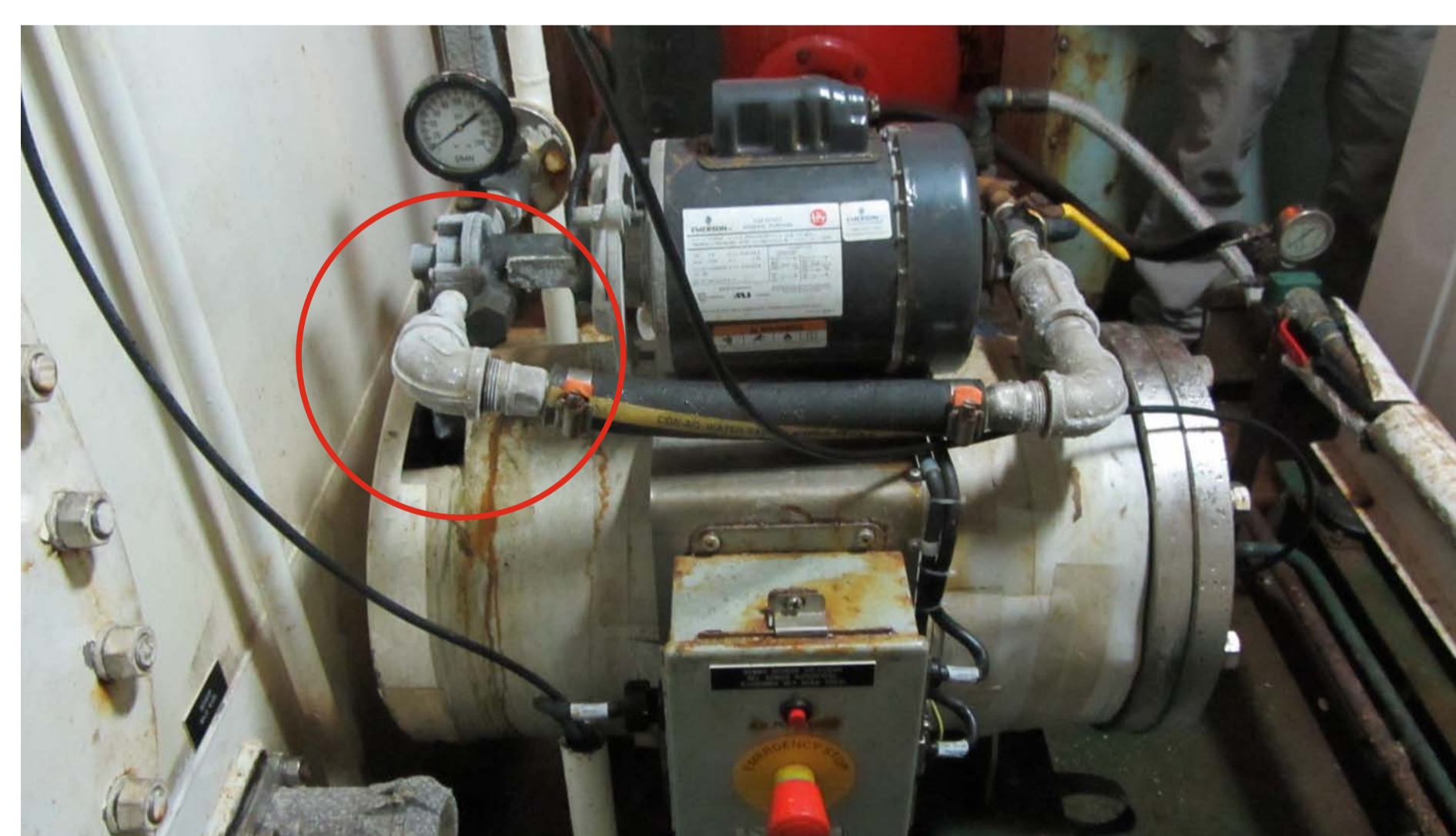
the water to flow constantly; this pump is installed inside the hold of the vessel, mainly to prevent the direct contact of the sensor with the ice that is frequently in work areas. Nevertheless, the adverse weather conditions in
