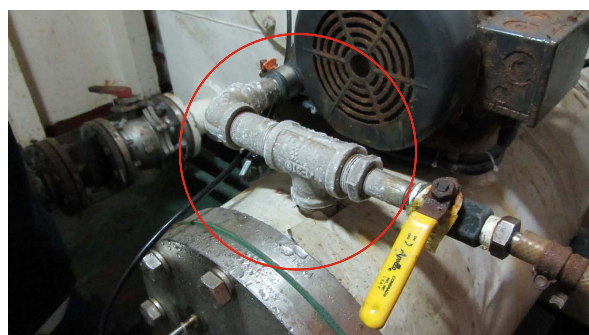
One of the major components of the multibeam system is the surface sound velocity sensor (SSV), whose aim is to monitor the sound velocity to 6.35 m depth every 2 seconds. This sensor is installed within a pump, which allows
